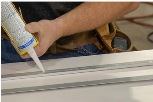
Adhere trim with only one of the approved GE Silicone products from page 2
